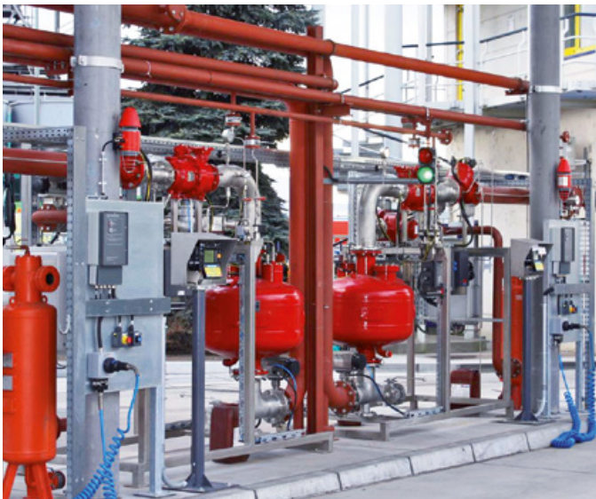
↑ CMS: Compact Metering Skid
